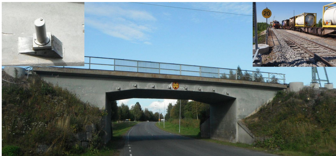
FIGURE 5.21 UPGRADED CONCRETE TROUGH BRIDGE BUILT IN 1959 IN HAPARANDA IN NORTHERN SWEDEN. IN 2012 THE BRIDGE WAS STRENGTHENED WITH EIGHT POST-STRESSED BARS INSTALLED IN HOLES DRILLED THROUGH THE SLAB (INSERT LEFT). ML-D1.1 (2013), (NILIMAA ET AL, 2013, 2014, 2015).
