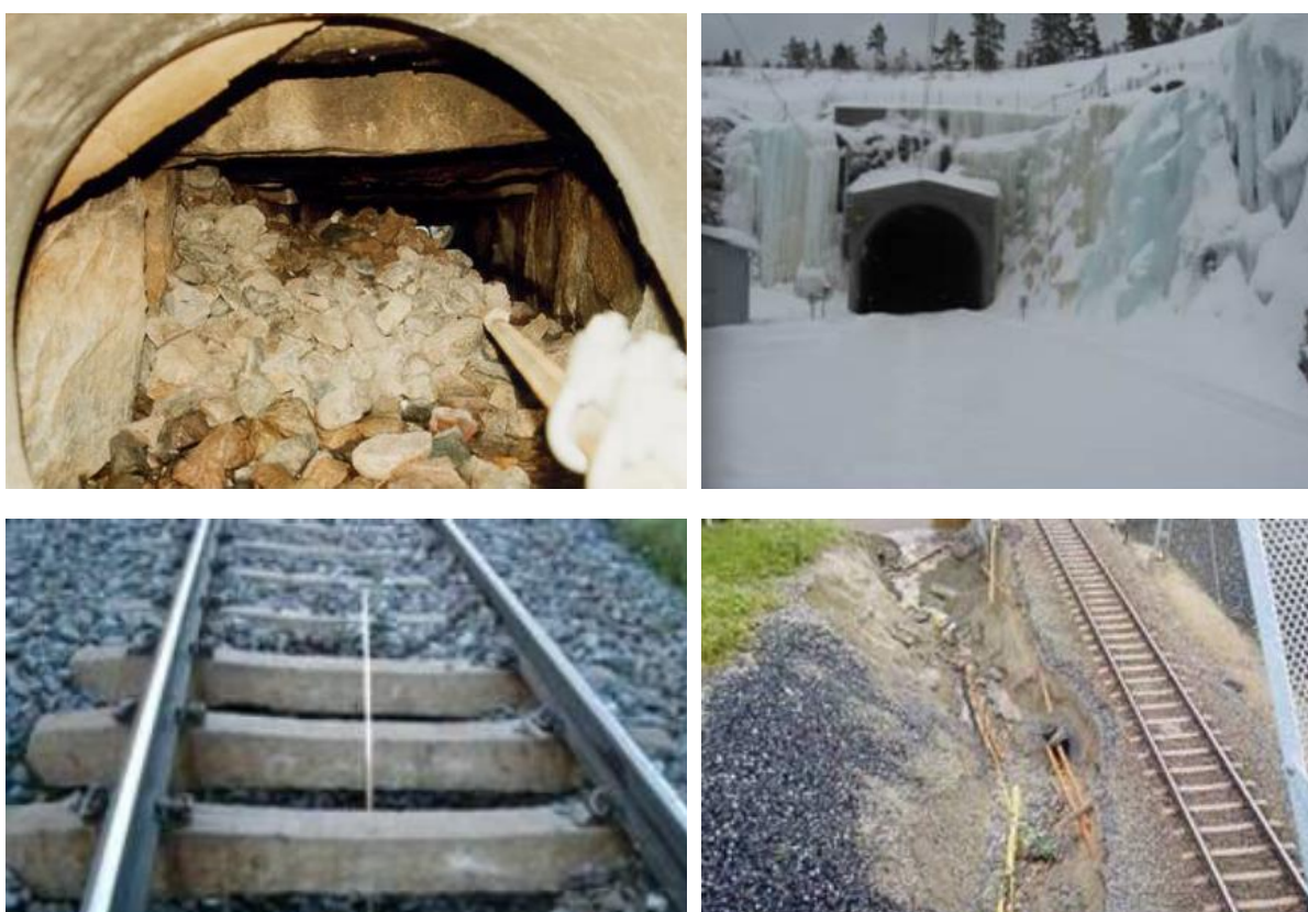
FIGURE 7.2. EXAMPLES OF DAMAGES IN CULVERTS (FROM TOP LEFT CLOCKWISE): (A) CRACKING AND DOWNFALL OF BANK MATERIAL; (B) ICE CLOGGING THE CULVERT; (C ) CRATER IN BANK DUE TO DOWNFALL OF MATERIAL INTO CULVERT; (D) EROSION ALONG BANK. TRVH AVVATTNING (2011).
