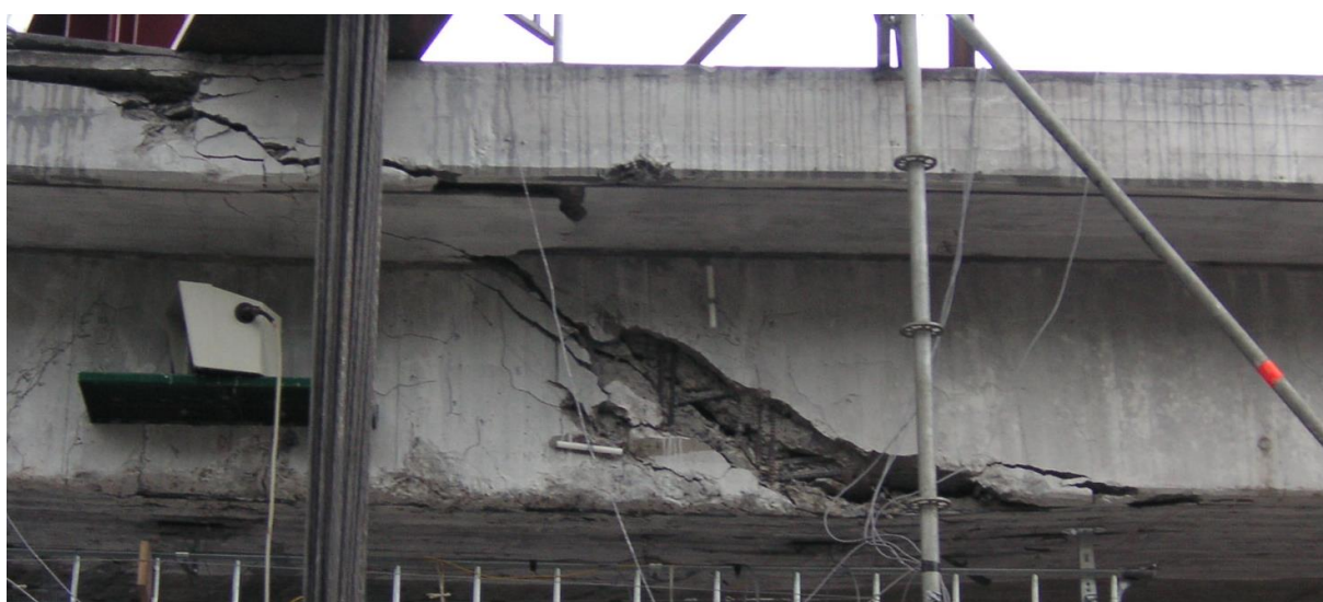
FIGURE 5.20 TEST TO FAILURE OF A STRENGTHENED TROUGH IN ÖRNKÖLDSVIK, 2006. TOP: OVERVIEW OF BRIDGE WITH EAST RAIL BANK CUT AWAY AND REPLACED BY A TEMPORARY ROAD TO SUBSTITUTE THE LANE UNDER THE BRIDGE SPAN BEING TESTED. BELOW: DETAIL OF FAILURE IN SOUTH BEAM CAUSED BY A COMBINATION OF STRESSES DUE TO BOND, SHEAR, BENDING AND TORSION. SB-D7.1 (2006), PUURULA ET AL (2012, 2014, 2015, 2016)).
