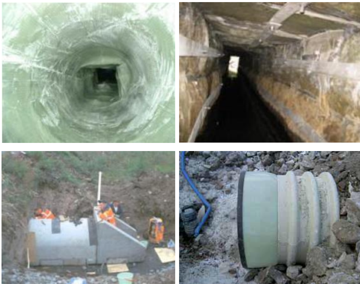
FIGURE 7.3. EXAMPLES OF MEASURES TO RESTORE CULVERTS (FROM TOP LEFT CLOCKWISE): (A) LINING WITH PLASTIC MATERIAL; (B) REPAIR OF JOINTS; (C) EXTENSION OF CULVERT; (D) CORRUGATED STEEL CULVERT REPAIRED WITH GLASS FIBRE LINING. THE LINING EXPANDS AT THE ENDS OF THE CULVERT AND STABILIZES THE EMBANKMENT. SÖDERGREN (2011), RAILCARE (2012), ML-D1.1 (2013).
