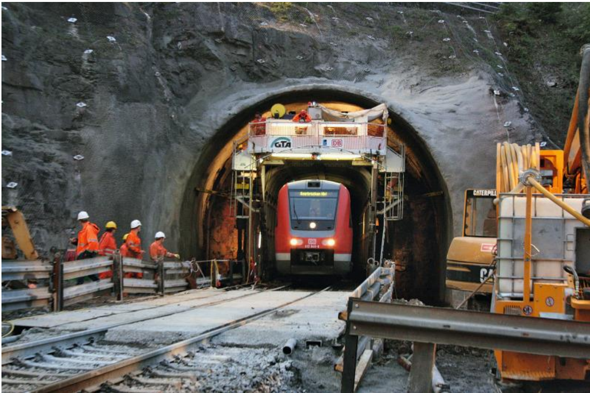
FIGURE 6.8. JÄHROD TUNNEL IN GERMANY BEING ENLARGED BY THE TUNNEL-IN-TUNNEL (TIT) METHOD, SIMON (2012).
