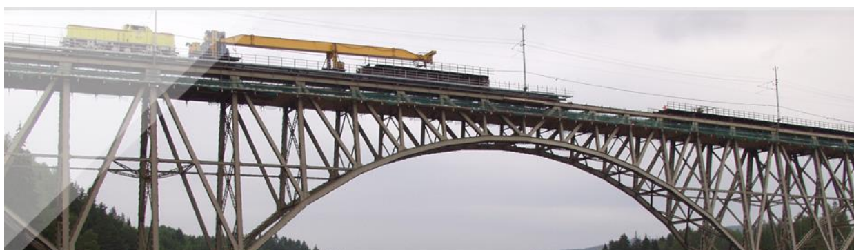
FIGURE 5.16 STEEL TRUSS ARCH WITH REPLACEMENT OF TOP STRUCTURE AT THE FORSMO BRIDGE. COLLIN ET AL (2010).
