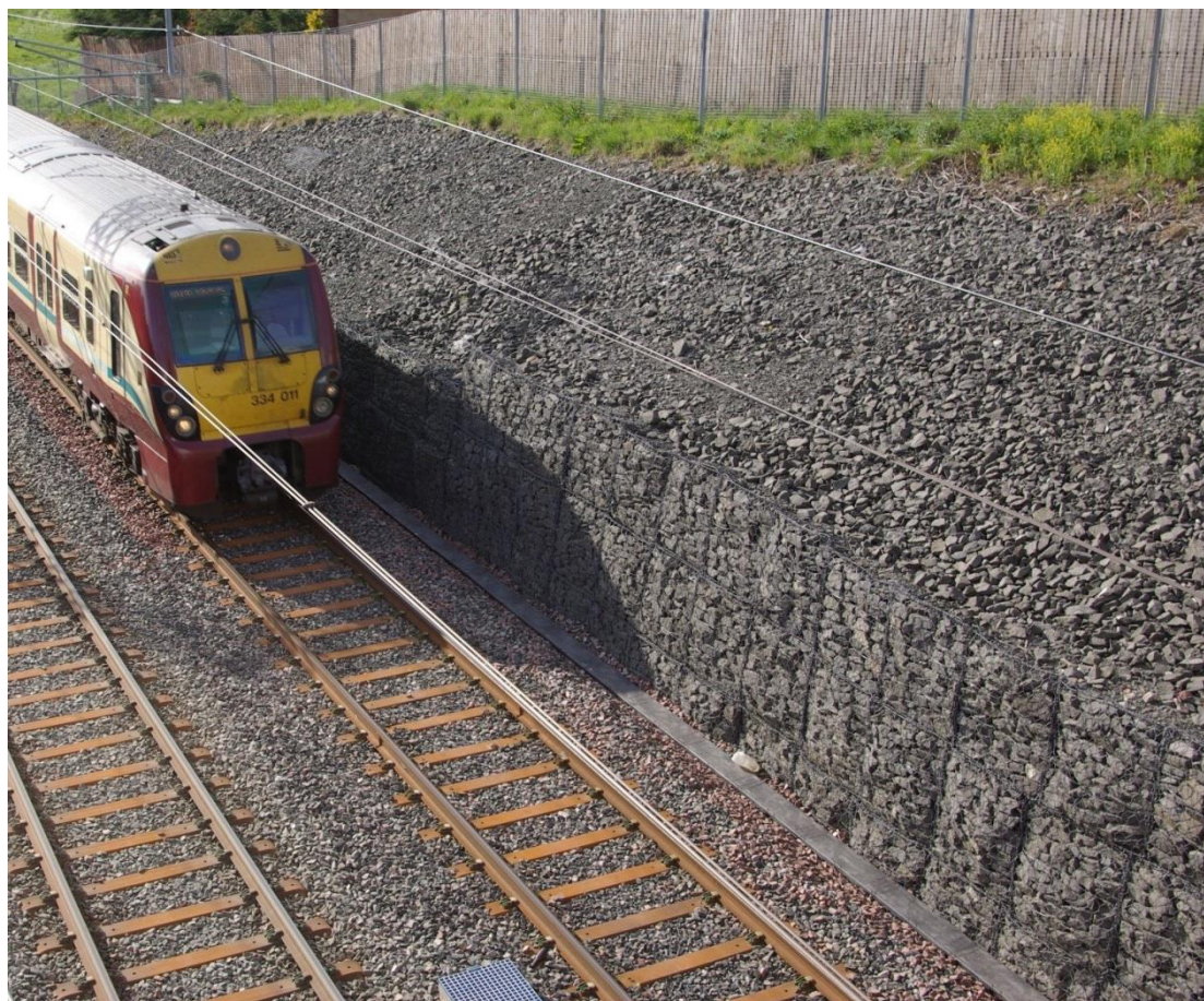
FIGURE 8.2. GABION RETAINING WALL AT THE NEW AIRDRIE TO BATHGATE PASSENGER RAIL LINK IN THE CENTRAL BELT OF SCOTLAND IS A LANDMARK PROJECT BY NETWORK RAIL TO WIDEN AND RE-OPEN A 24KM LINE CLOSED OVER 50 YEARS AGO. GABION (2015).
