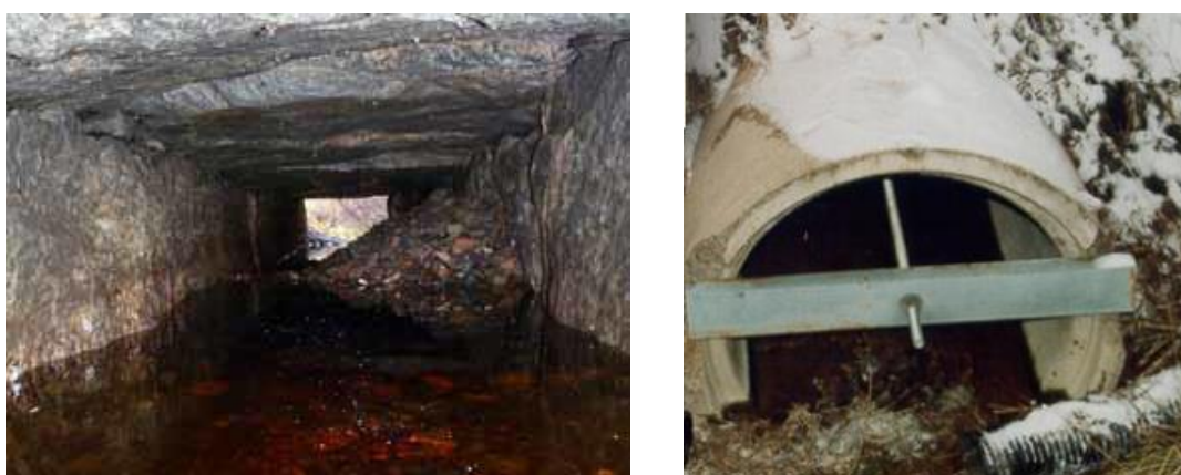
FIGURE 7.4. LEFT: OLD STONE CULVERT WHERE THE BOULDERS HAVE SEPARATED AND SAND AND MUD HAVE POURED DOWN. RIGHT: A CULVERT IS KEPT TOGETHER BY POST-TENSIONING OF STEEL BARS SJÖBERG ET AL (1998), TRVH AVVATTNING (2011).
