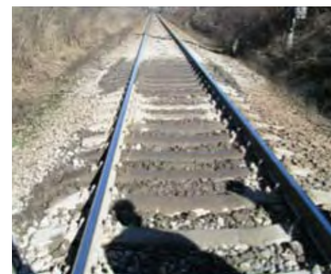
Figure 4.2.3-1: Track with drainage defects before reparation
