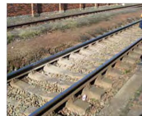
Figure 4.2.3-2: Station track with clear drainage defects
