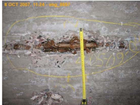
A picture above is from the special inspection showed a bar that had no grouting and some corrosion.
