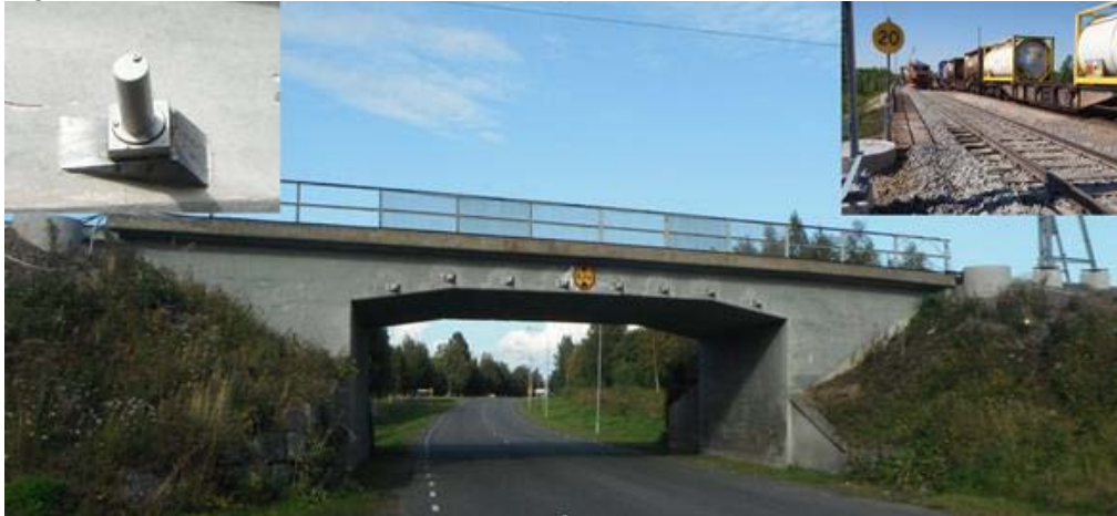
Figure D-x The Haparanda Railway Bridge (3500-2033-1, km1309+609) was strengthened in the summer of 2012. Eight transverse prestressing bars were installed at mid-height of the slab (left insert) and posttensioned to upgrade the axle load capacity of the railway line from 25 to 30 ton.
