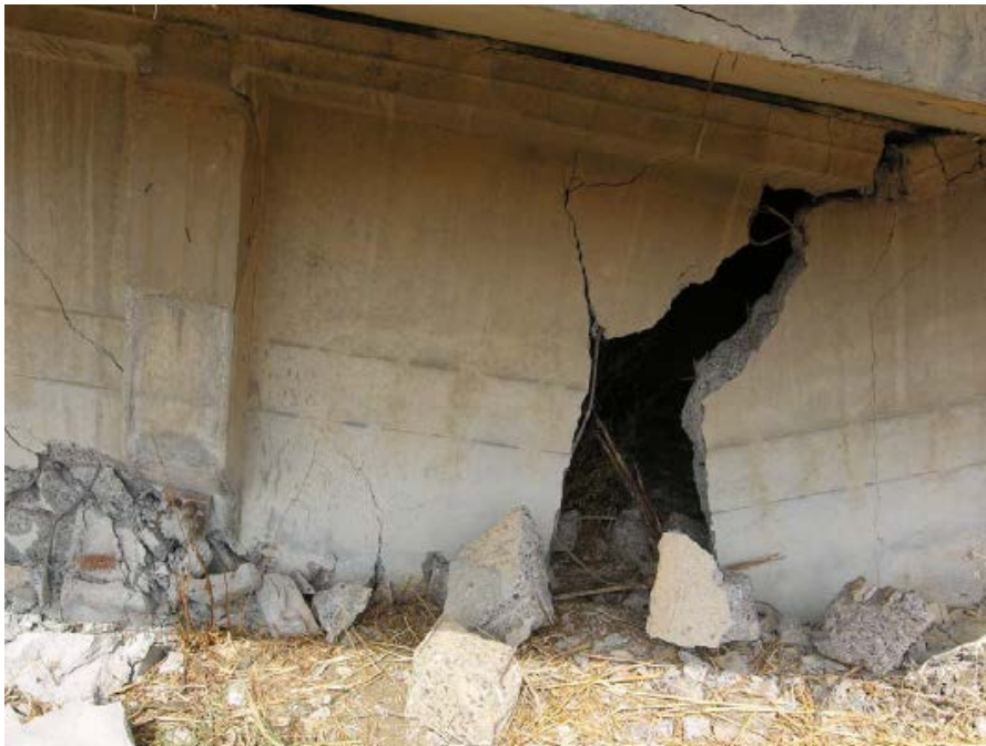
Figure 3.7. Mid-span fracture of prefabricated prestressed beams in Sicily in 2014, Anania et al (2018).
