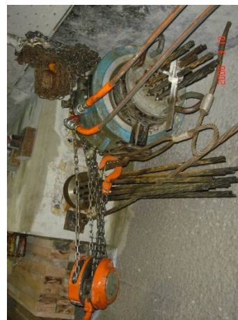
Prestressing of cable at top - "live end". "Dead end" for cable at bottom.
