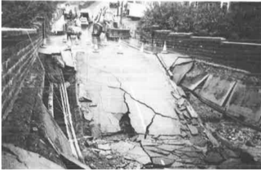
Figure 3.6. Collapse of bridge in Wales 1985. Woodward (1989).
