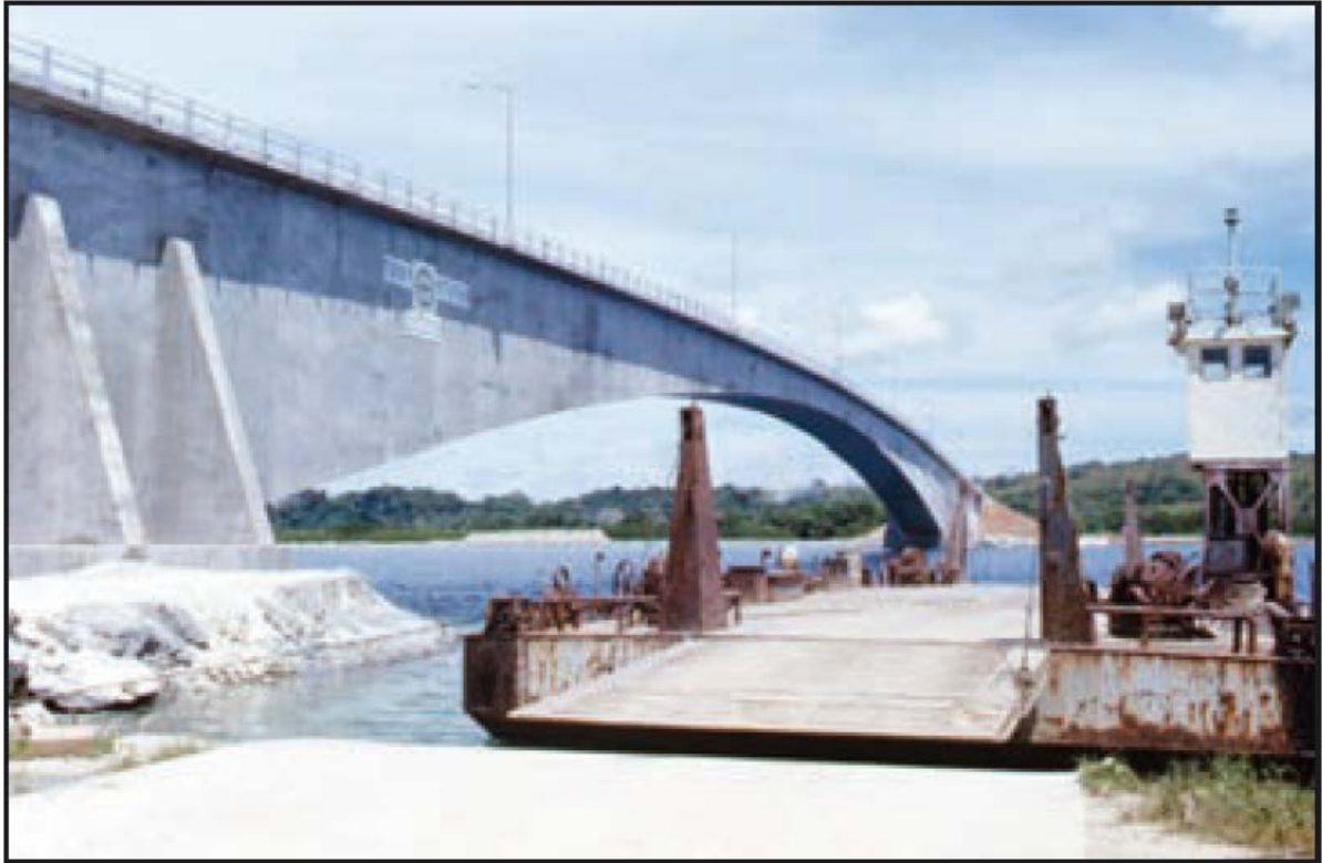
Figure 6.4 The 249 m span of the prestressed Koror bridge (and the ferry it replaced) before failure in 1996 due to creep and relaxation, Tang (2014).
